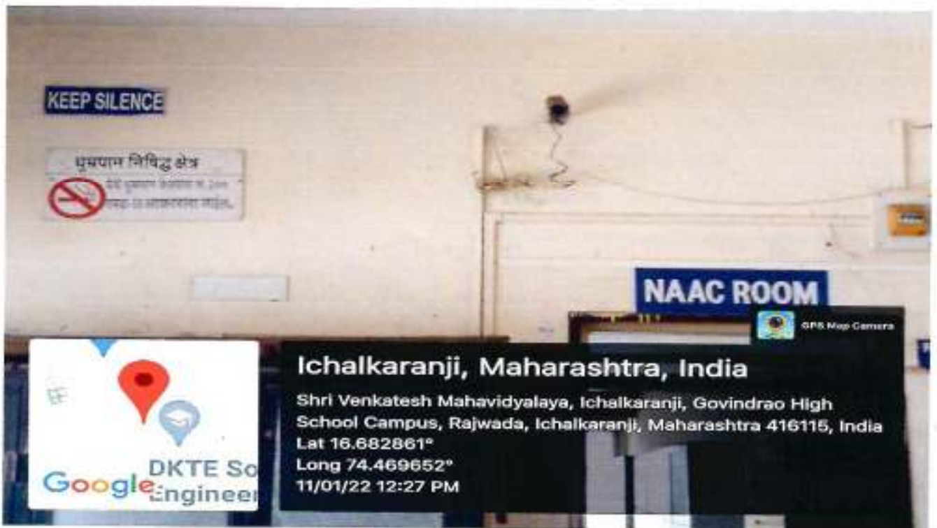
CCTV Camera at NAAC Room
