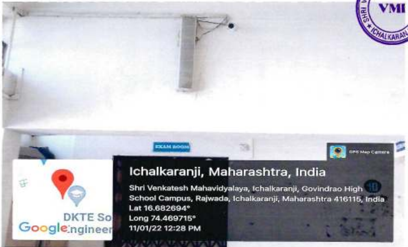
CCTV Camera at Exam Room
